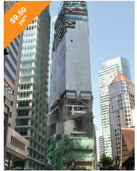
18 Robinson Road Robinson Road
